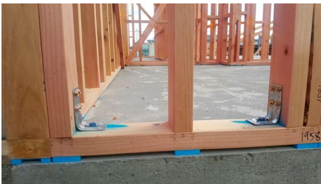
Bracing element showing “Proprietary” hold down bolt/bracket.
